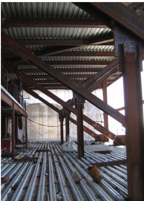
Figure 2- Outrigger bracing on mechanical floor, courtesy of Thornton Tomasetti
